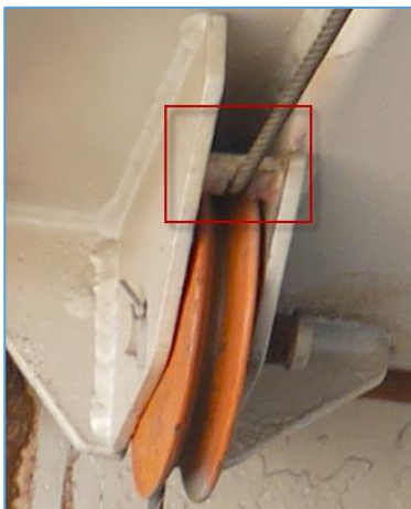
← 3. Photo of static line (transverse deck stabilizing cable) that is misrouted below the spacer (rubbing on spacer).
