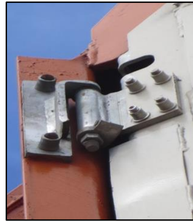
Broken Hinge at Top of Door
