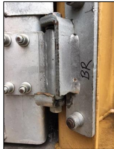
Broken Hinge at Bottom of Door
